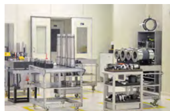
Ultra Clean room
